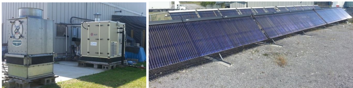
Figure 29. (a) Liquid desiccant air handling unit and cooling tower as installed at Queen's University (b) Photo of the solar thermal collector array [4]
