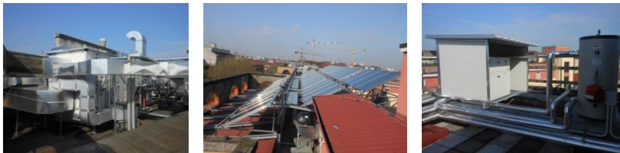
Figure 52: Photos of DEC AHU, solar collector field and the electric heat pump
